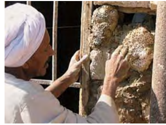
Photo 2 Research on the architecture and restoration of coral buildings in the Sinai Peninsula, Egypt.
